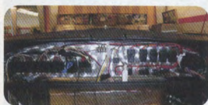
Behind the dash panel is where the electrical relays and terminal blocks are mounted neatly in groups. To the left are the power windows, center are the door poppers, and to the left are the Street & Performance EFI engine management relays.
