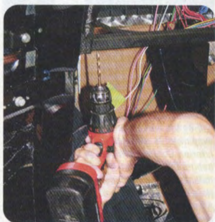
Robert drilled two mounting holes in the bottom surface of the steel tube that supports the painted dash panel.
